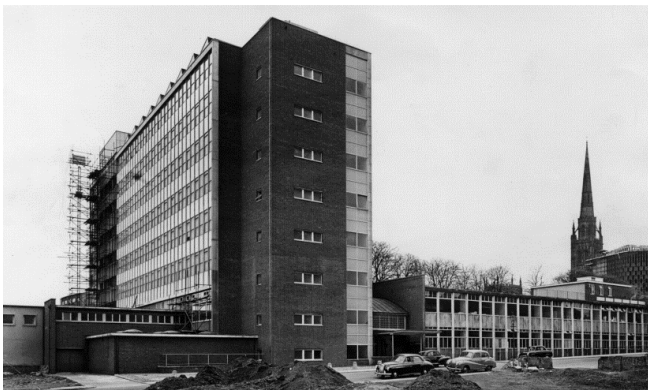
Figure 3. Final construction phase of the former Lanchester College of Technology in the 1960's known today as The Charles Ward building.
